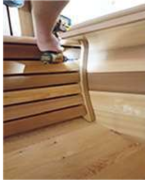
Screw the enclosures and the seat benches to the front wall with 2 ½" (64mm) screws. Screw between the slats to ensure screws are less visible
